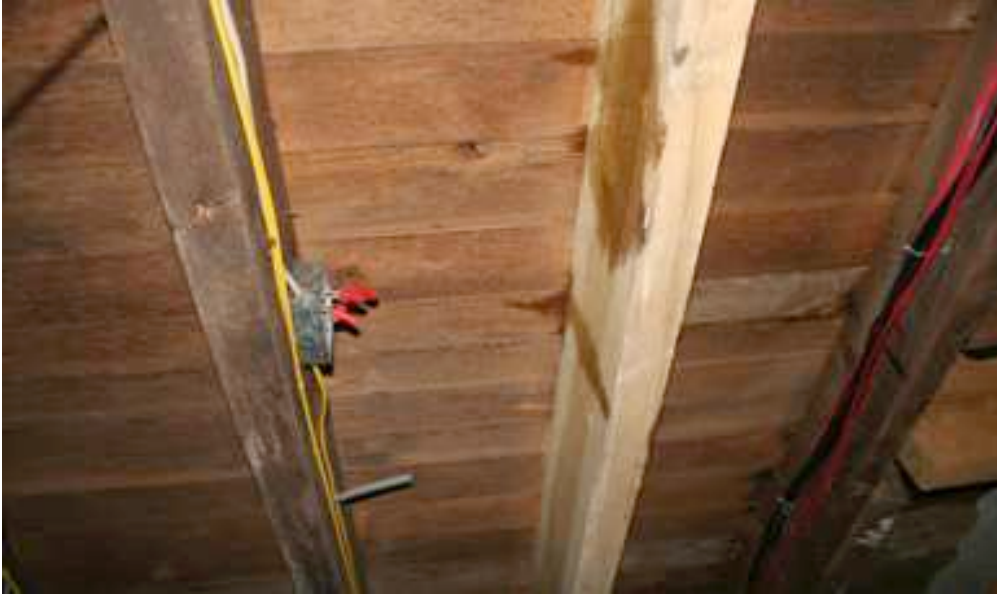
Figure 8. Basement ceiling of Daniel Lady Farm below stains on floor above. Note the capillary action causing absorption of water from the prior flushing procedures above.
