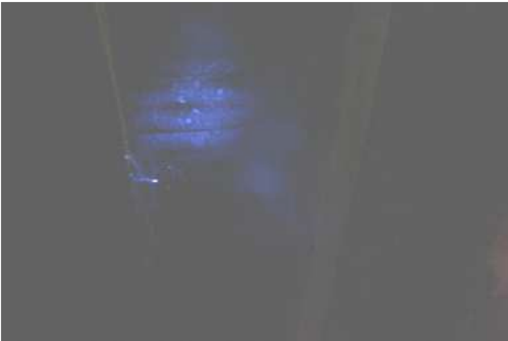
Figure 9. Chemiluminescent reaction observed on the basement ceiling. No reaction was observed in the tongue and groove seams or on the replaced beam.
